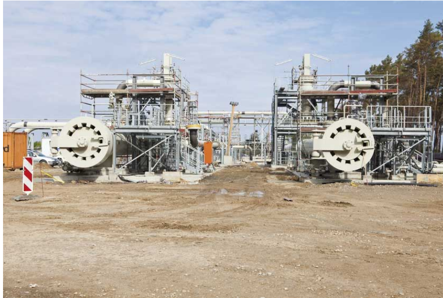
Nordstream PIG Launching and Receiving Station
